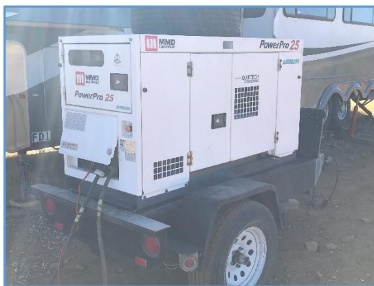
One of the six generators used at the North Fire ICP. Note that this unit was placed less than five feet from the RV trailer.
